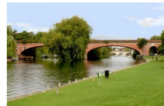
Maidenhead Railroad Bridge designed & built by I.K. Brunel in 1838 and still in use
