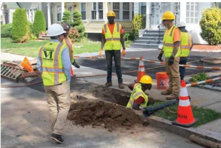
Crews have replaced more than 22k lead service lines throughout the city.
