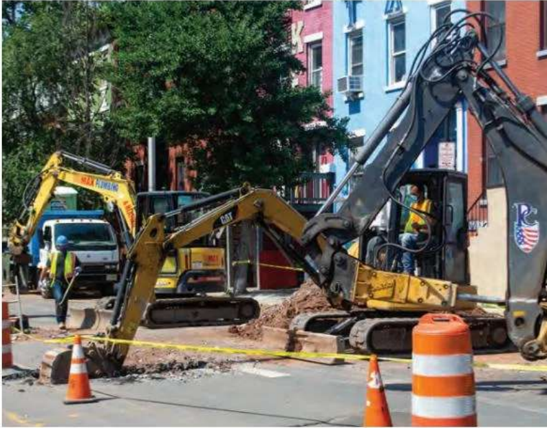
Crews made up of Minority/Women Owned Business Enterprises (MWBE) remove lead service lines. The City is scheduled to complete the Lead Service Line Replacement Program this fall.
