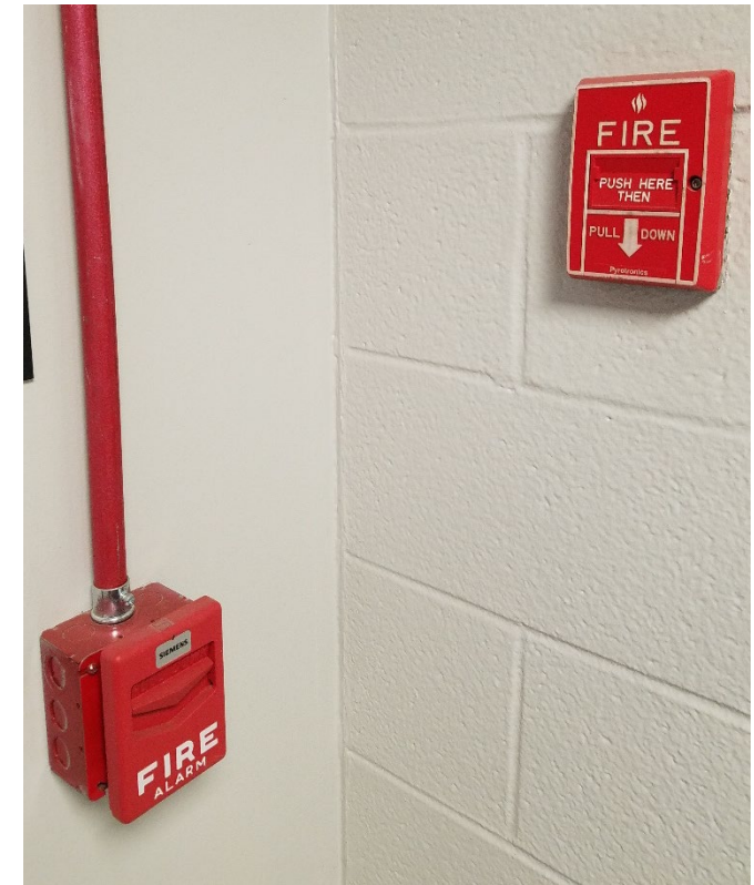
Old and New Pull Stations Operating Side-by-Side
