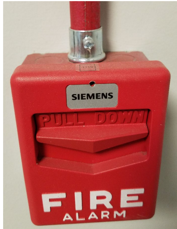
New Pull Station
