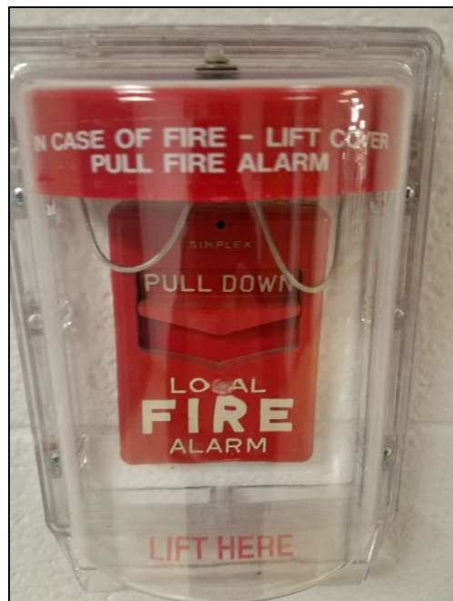
Pull Stations with Protective Covers
