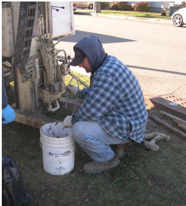
Groundwater sampling from a screen point driven in the ground by a geoprobe.
